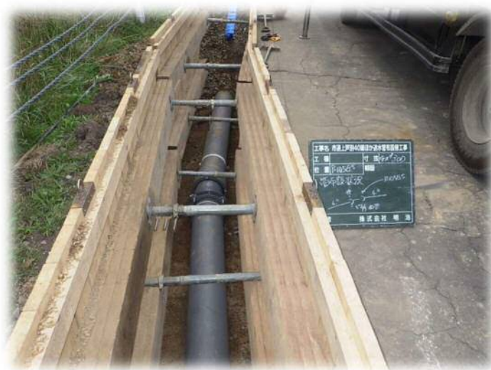
[管路の耐震化]
